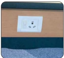
Power Switch Socket
